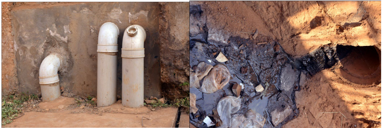
On the left (above) are pipes from Leading Lines Enterprises Ltd connecting to the big pipe on the right through which waste from the factory is emitted to the community and Kiyanja / Kirokole wetland.
