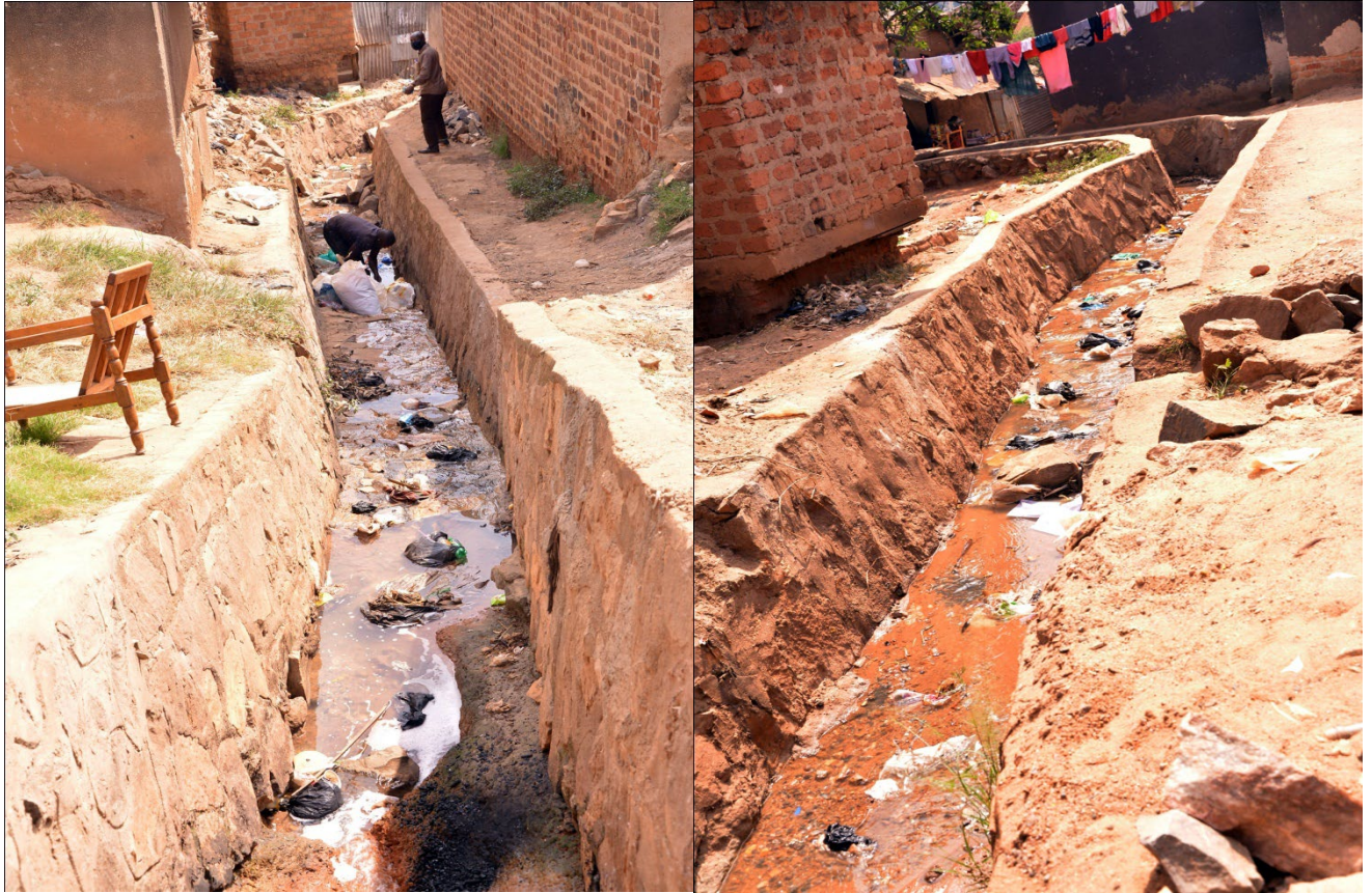
The above are two different parts of one drainage trench which community members said carries dirty liquid waste from Riham Factory every day. They suspect that the waste includes sewage from the factory.
